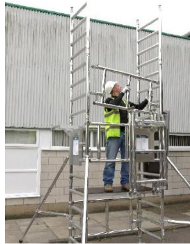
23. Retrieve a side guardrail frame from the front assembly bracket and locate it as shown.
