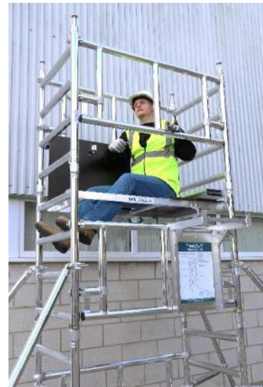
13. Fit 2 guardrail frames, with the top hook (facing outwards) set above the top rung of the frame.
