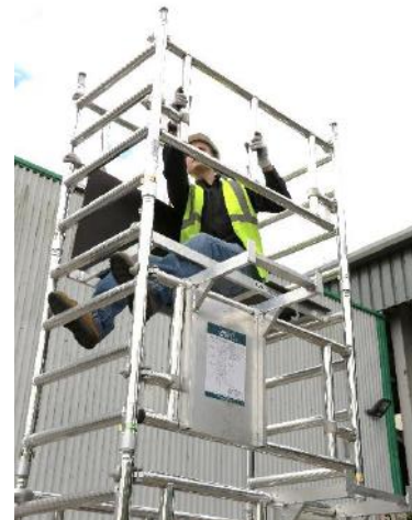
28. Fit 2 guardrail frames, with the top hook (facing outwards) set above the top rung of the frame.
