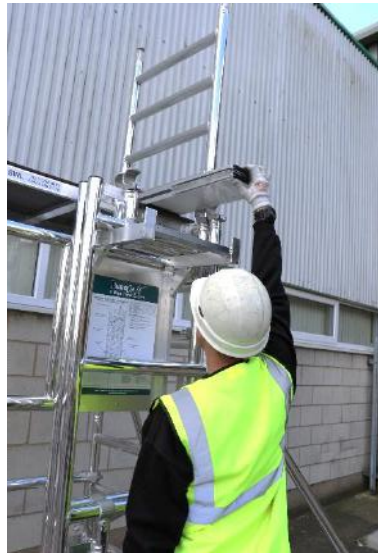
12. Relocate the toeboard assembly from the lower platform to the higher level, ensuring that it is positioned on the plain section of the platform as shown.
