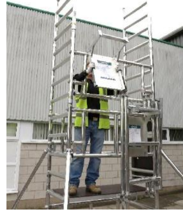
24. Relocate the side "empty" assembly bracket on the front of the tower (top rung of the tallest guardrail frame as shown)
